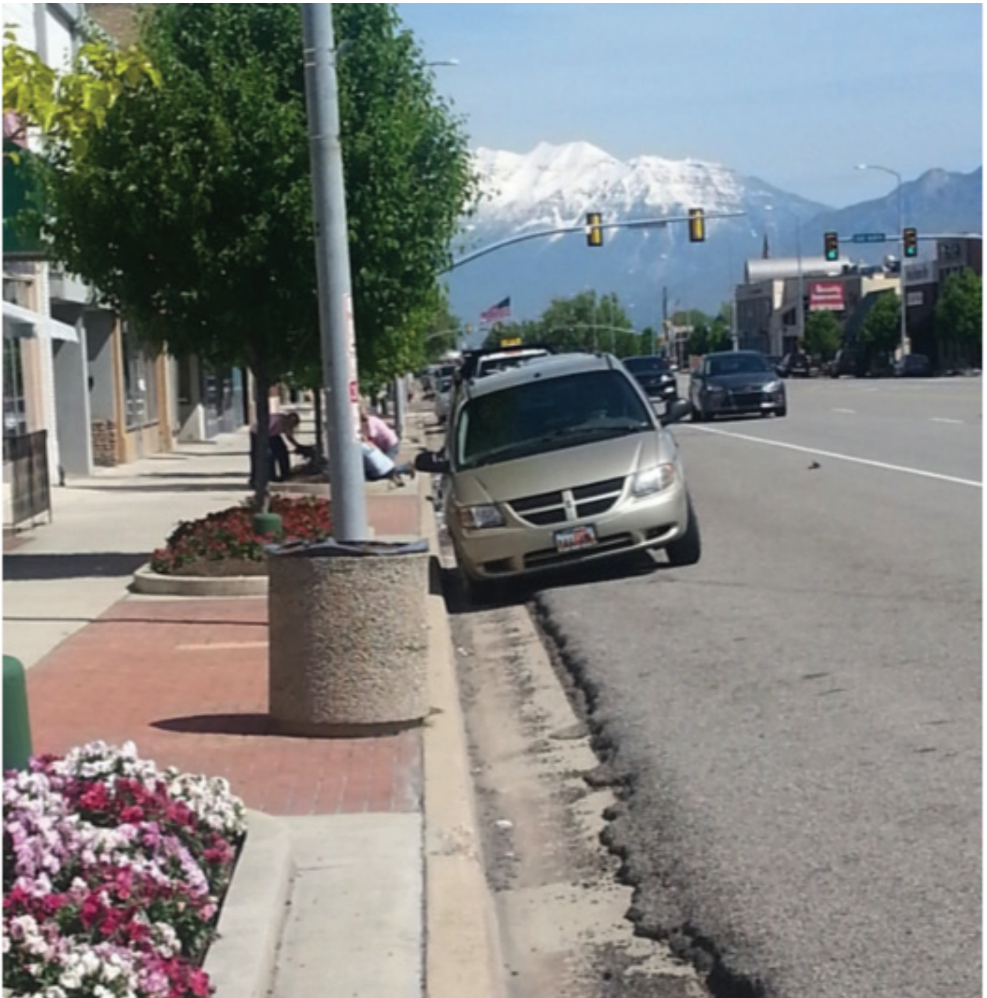
Asphalt buildup on Main Street
